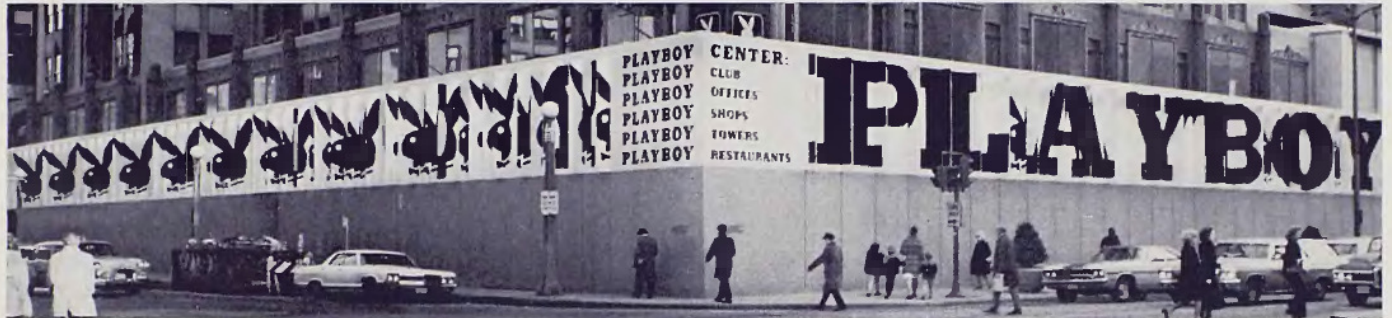
Arcade-style ground floor plus new Playboy Club is shaping up behind barricade.
